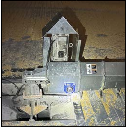
Center Pivot, Motor and Sump No main chain adjustment needed.
