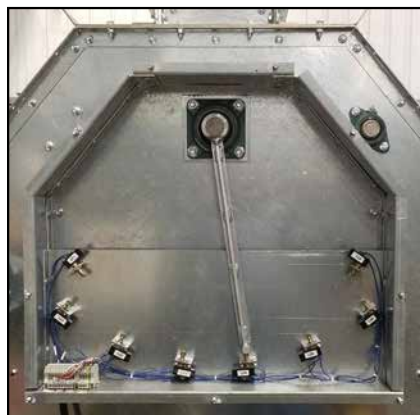
Electric Swing Distributor (with cover removed)
